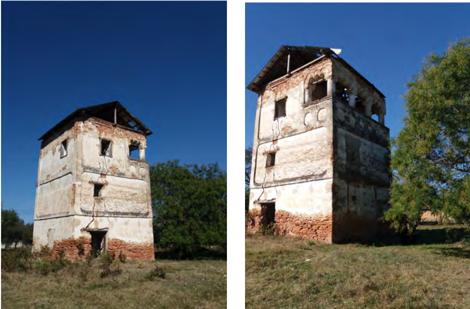
Fig. 14. Cula (tower dwelling) Ciobă-Chintescu from Şiacu, Slivileşti commune, Gorj County (photo A. Rustoiu).
