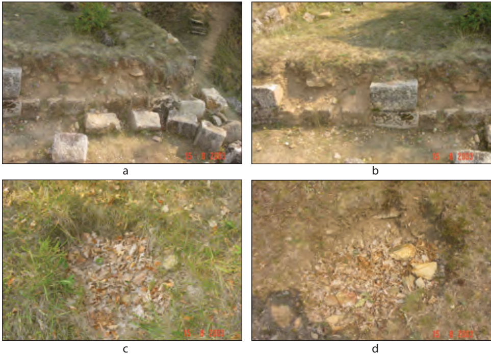
Figure 4. Photos taken in August 2003: the wall of the dwelling-tower collapsed (a-b); pits dug by poachers (c-d) (photo by R. Totoianu).
